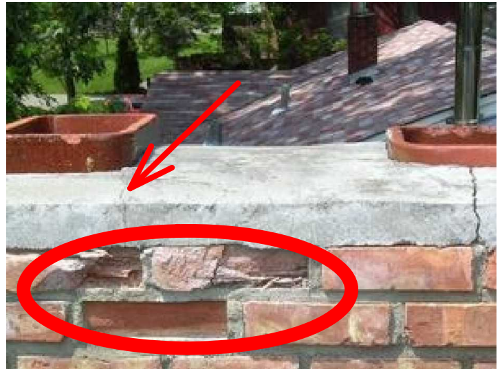
Cracked chimney cap and spalling bricks.
