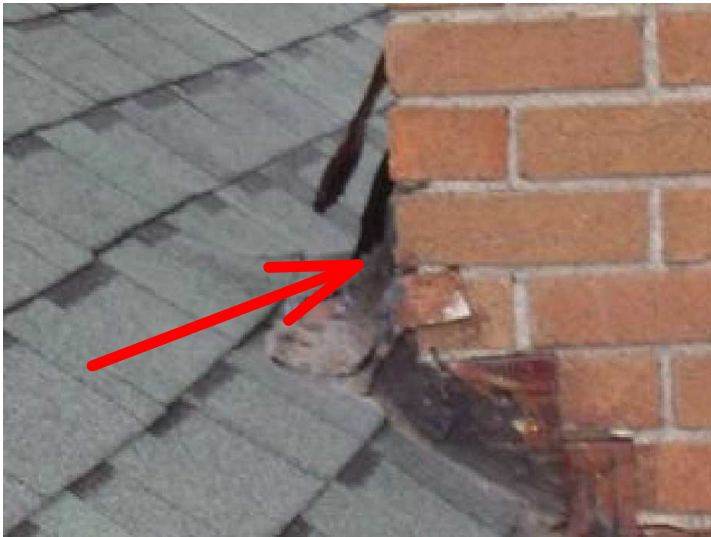
Loose chimney flashing
