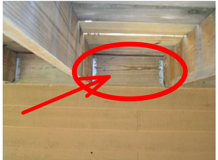
Missing lag bolts on a deck ledger board.
