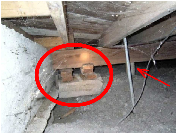
Improperly supported and sagging main beam.
