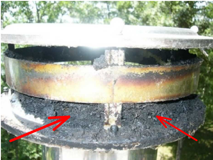
Creosote caked chimney flue poses a fire hazard.
