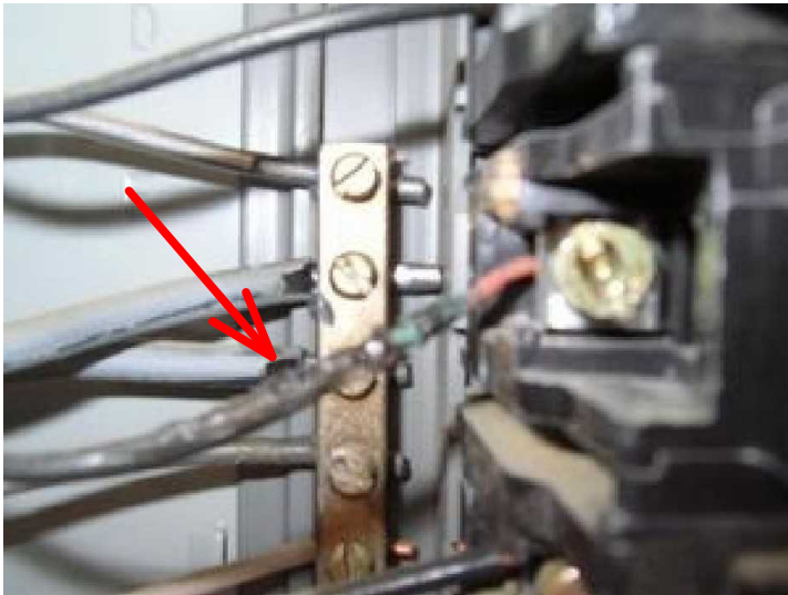
Overheated electrical wires.
