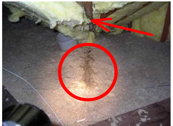
Leaking roof valley.
