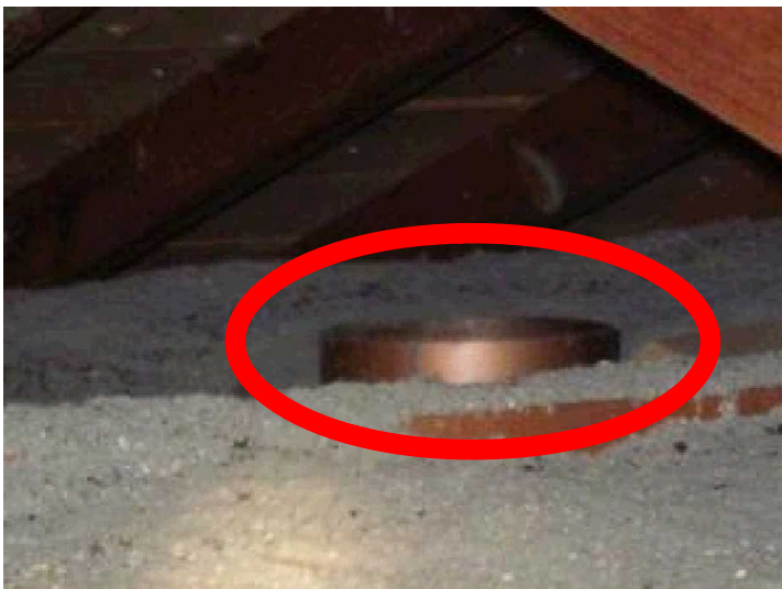
The kitchen exhaust is ducting into the attic.
