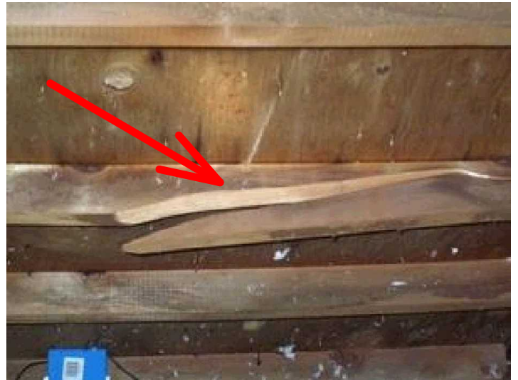
Cracked roof rafter.
