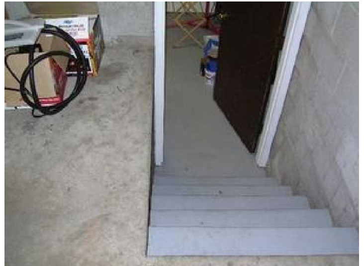
Missing hand rails.
