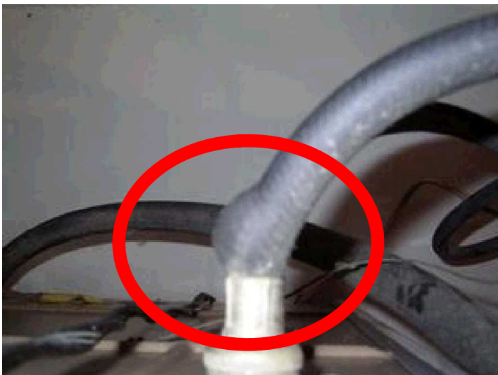
When was the last time you checked your washing machine supply lines.
