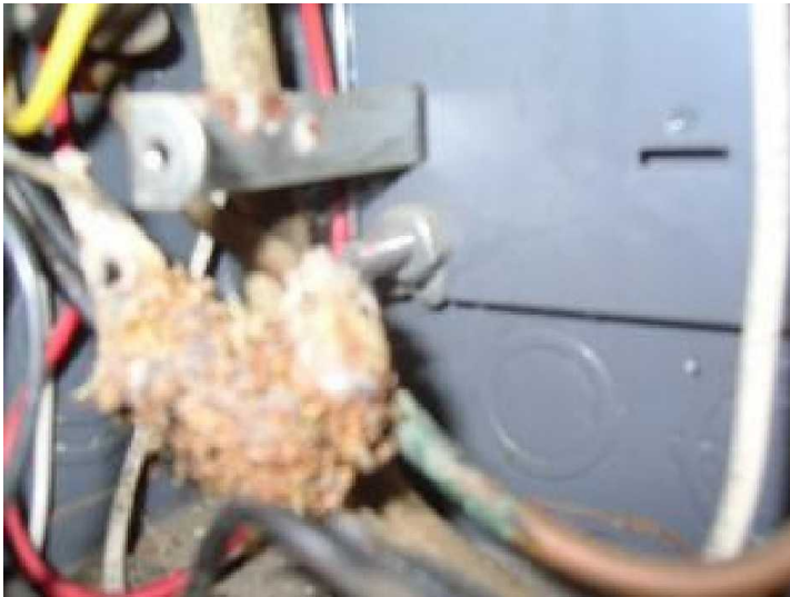
Missing knock outs allow rodent entry
